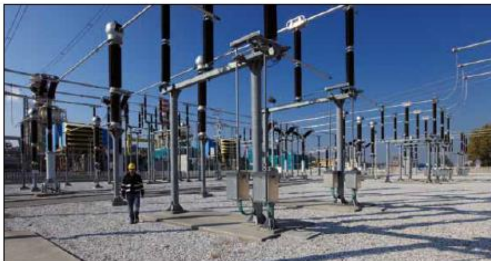
► Security of supply is a basic goal of the power generation sector.
