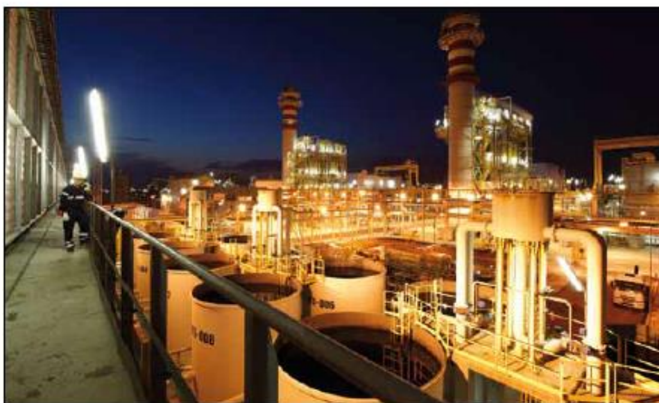
◆ Power plants using CCGTs such as this one in Ferrara, Italy are efficient and flexible.
